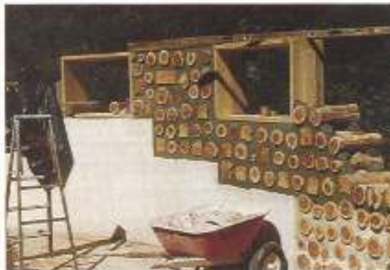
ABOVE: Stockadestyle cabins turn logs on their end and look like frontier forts. They also allow the use of shorter logs to fashion the walls.
